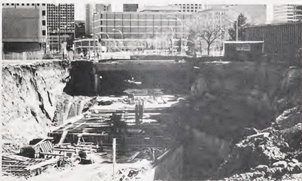
Plate 47. (Author's Photograph) Cut and Cover Construction at North End of Churchill Station, 1977
